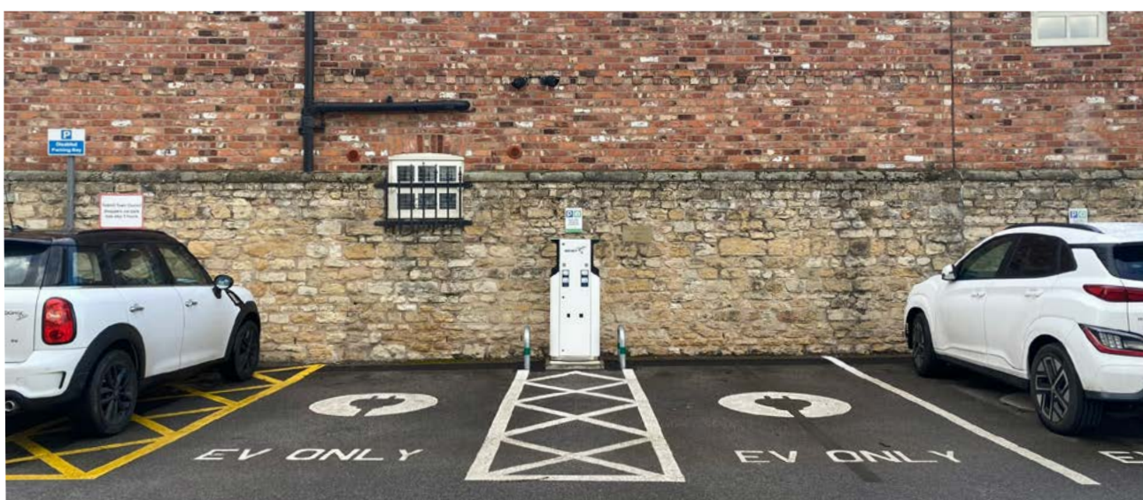
Figure 218: Public electric vehicle charging points in Tickhill, South Yorkshire.
